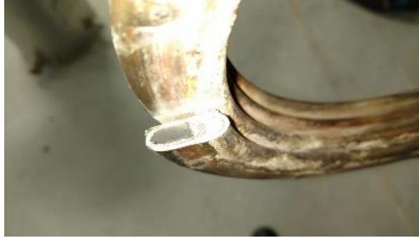
Figure 2 - watertube failure after one year of service
