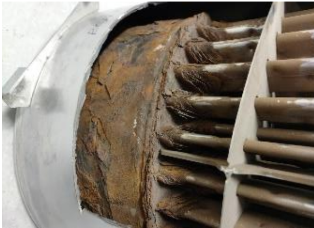
Figure 3 - less than one year old firetube exchanger (courtesy of NTI Boilers)
